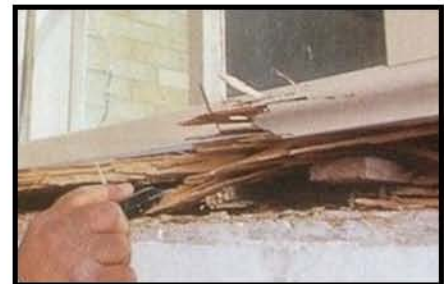
Formosan Subterranean Termite—Damage
